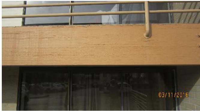
Wood facade on the patios, ceiling panels above the patios and wood trim. 8,344 lin. ft.
